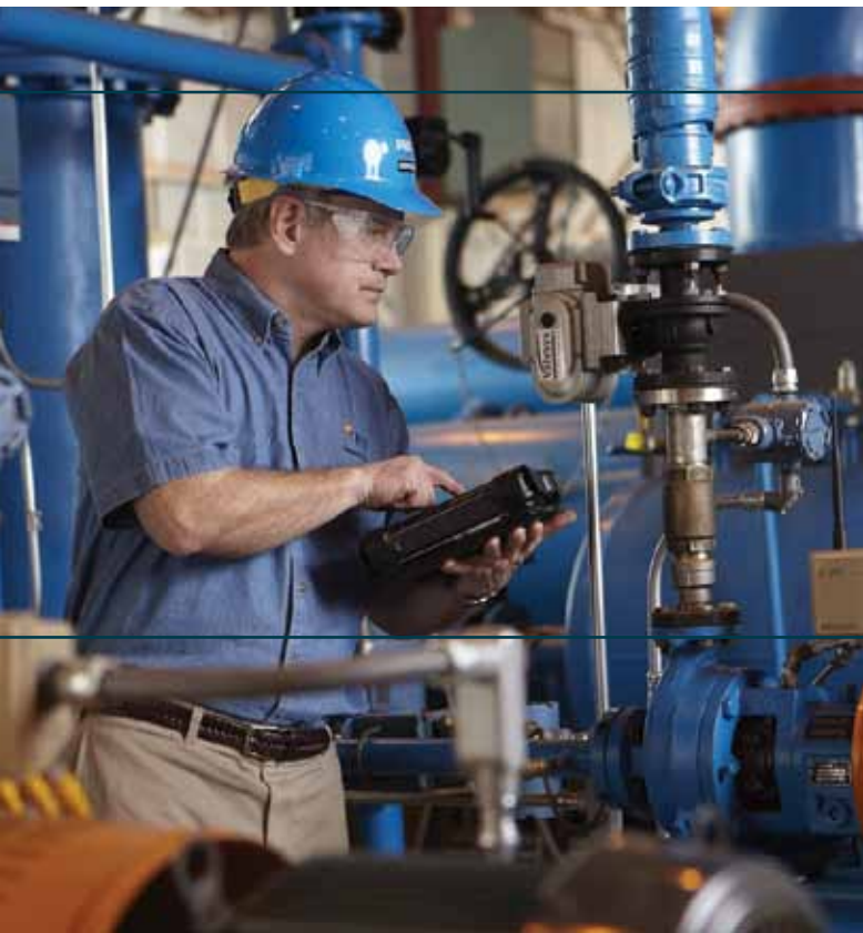
An ITT specialist capturing equipment data directly into ProWare, a proprietary computer reliability software program.
